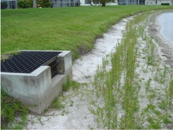
Fig. 2 An Example of Bank Scour
