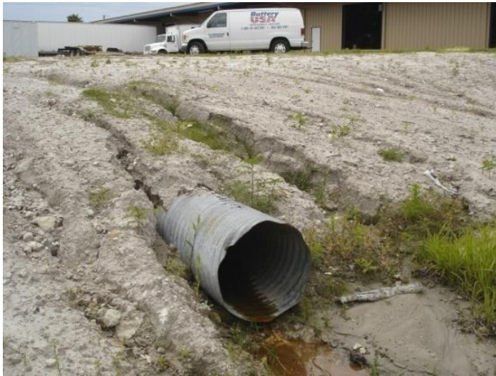
Fig. 1 An Example of Bank Erosion
